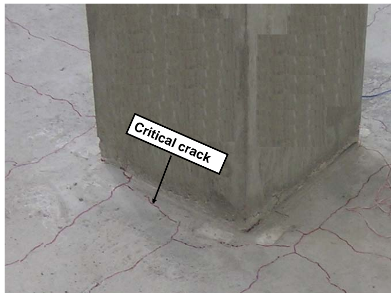
Figure 4.6 Critical crack in Specimen LR ST G0.5 (South axis)
