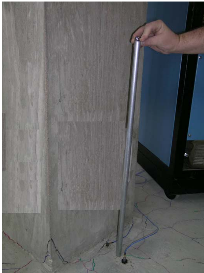
Figure 6.6 Crack depth measurements using a steel pipe to drop the ball at the precise position of impact
